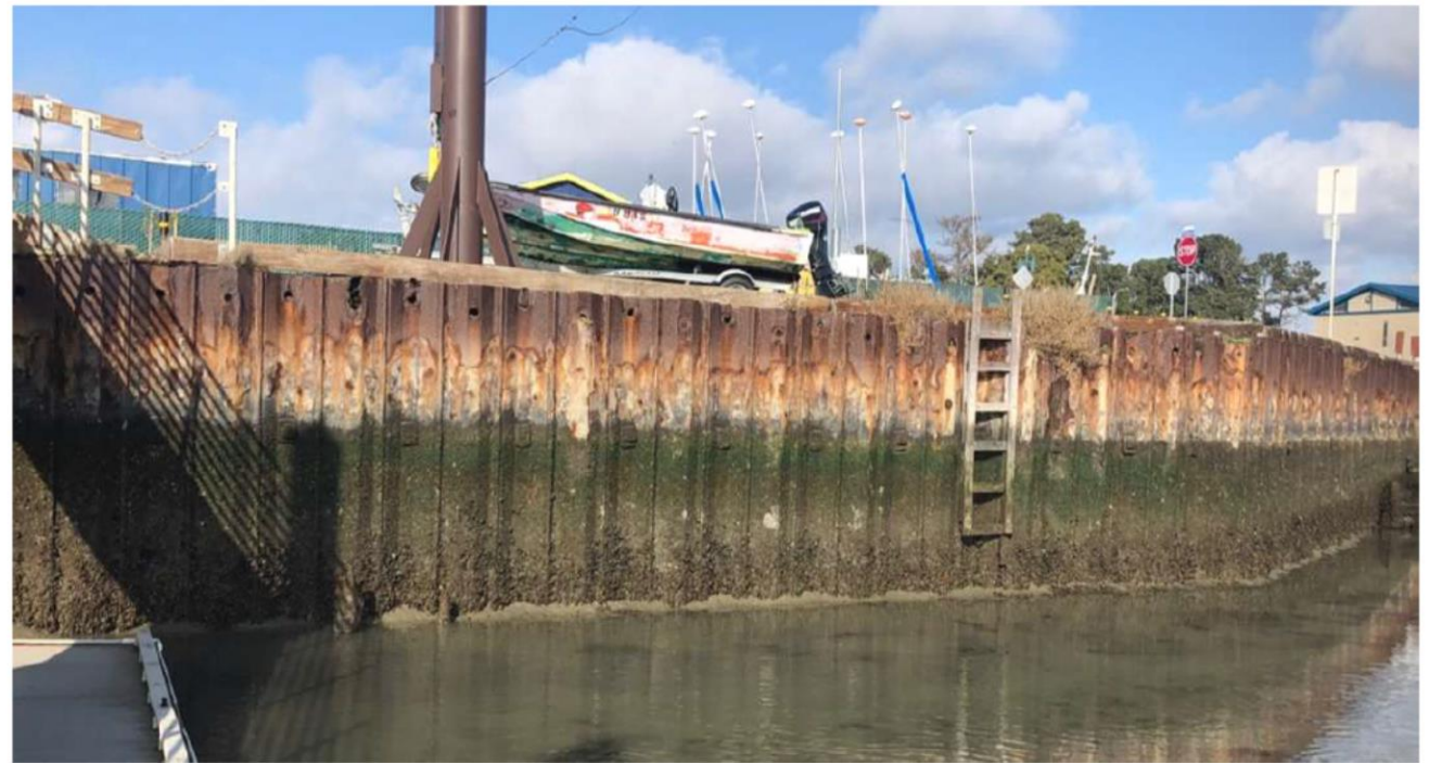
South Sailing Cove Seawall. Note the heavily corroded steel of the sheet piles.
