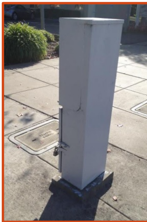
Example of a safety enclosure in the public right-of-way in Berkeley; Pilot applicants have the option of using a similar enclosure for charging stations
