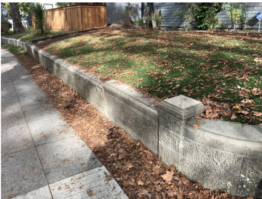
Detail of cast stone site wall along south and east sides of property; near corner, looking northwest.
