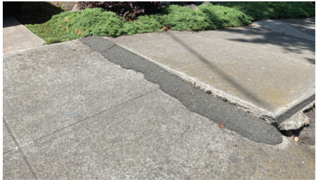
Before: Damaged sidewalks and long repair waitlist
