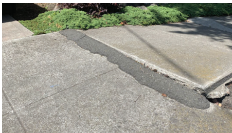
Before: Damaged sidewalks and long repair waitlist
