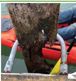
Before: Decayed timber piles
