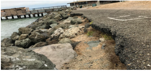
Before: Corroded, deteriorating seawall
