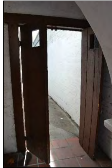
Figure 23. Paired door opening to the pedestrian alley between the two adjacent buildings Source: ARG, November 2024
