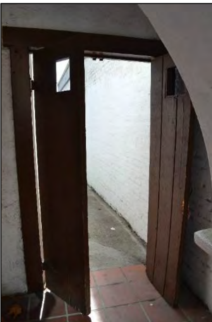
Pairing of wood doors at the west end of 2506 Haste Street's north façade, which leads into the rear pedestrian alley
