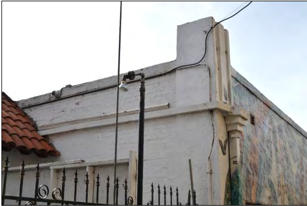
Northeast corner pier and exposed brick at the east façade of 2455 Telegraph Avenue
