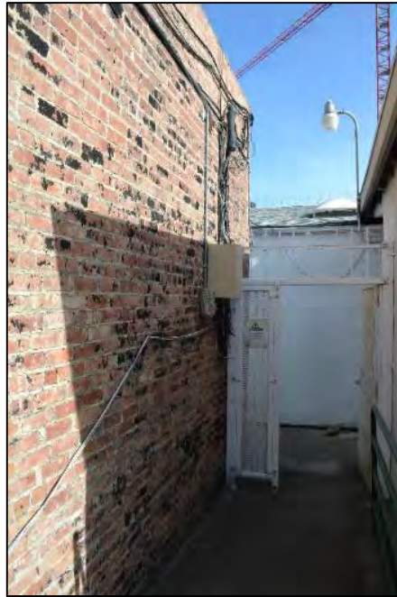
Rear pedestrian alley, viewed facing east; the south wall of 2455 Telegraph Avenue is at left, and the west wall of 2506 Haste Street is right of center
