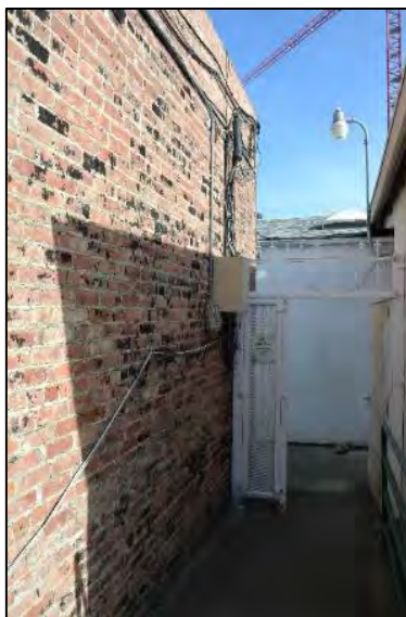
Figure 16. Unpainted brick exposed at the east end of the south façade, viewed facing east from the rear alley Source: ARG, November 2024
