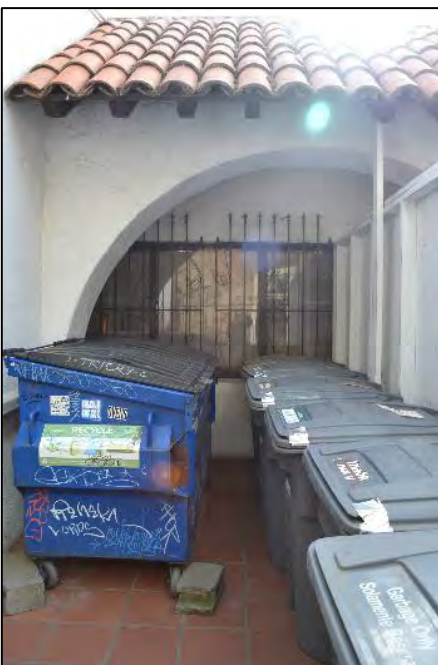
Service area near the west end of 2506 Haste Street's north façade, featuring an arched opening
