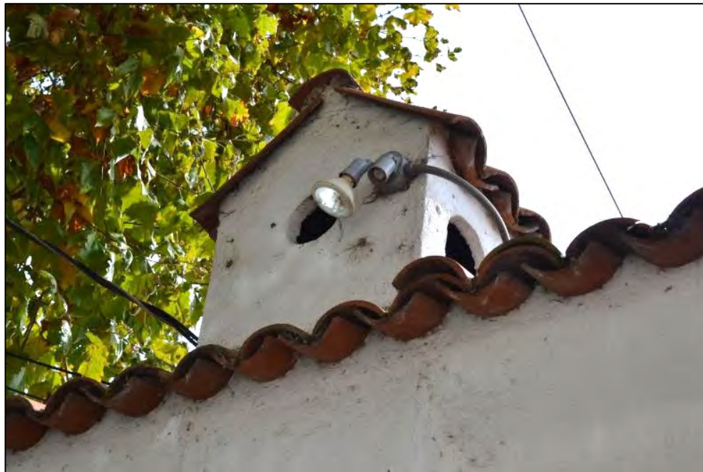
Tiled chimney cap above the roofline at the north façade of 2506 Haste Street
