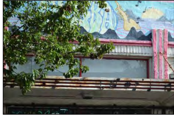
Figure 7. Detail view of clerestory windows and the molded stringcourse above the marquee Source: ARG, November 2024
