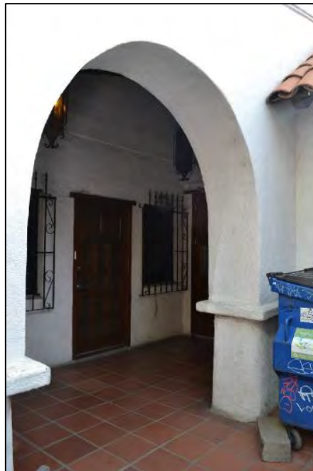
Door and windows within the vestibule at the center of 2506 Haste Street's north façade, viewed facing southeast
