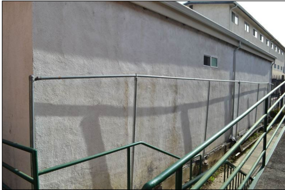
West wall of the south addition of 2506 Haste Street, viewed facing southeast from the rear pedestrian alley
