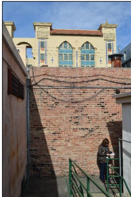
Exposed brick at the south wall of 2455 Telegraph Avenue, viewed facing north from the rear pedestrian alley
