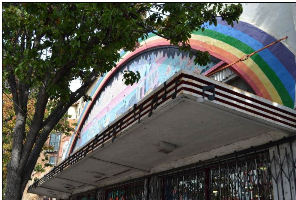
Detail of marquee spanning the front façade and arched frame, viewed facing northeast
