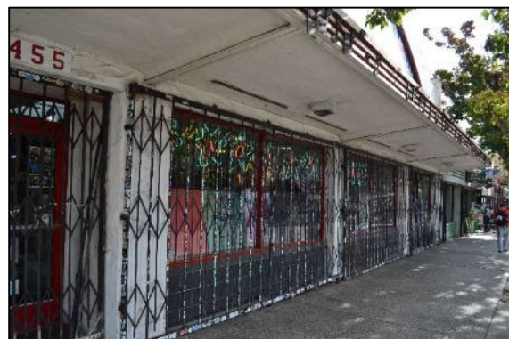
Figure 5. Remaining three bays at the primary façade, each of which contains a pairing of display windows Source: ARG, November 2024
