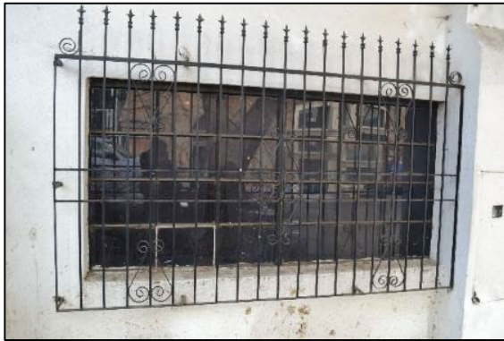
Figure 18. Window with security grate near the east end of 2506 Haste Street's north façade Source: ARG, November 2024
