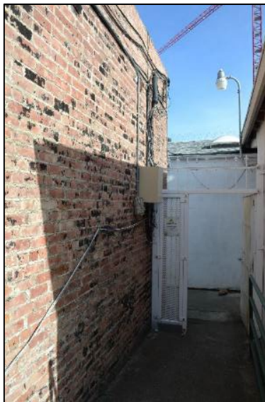
Figure 16. Unpainted brick exposed at the east end of the south façade, viewed facing east from the rear alley Source: ARG, November 2024
