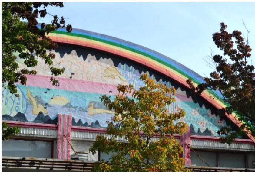
Figure 8. Painted mural within the arched parapet at the front façade, viewed facing east Source: ARG, November 2024
