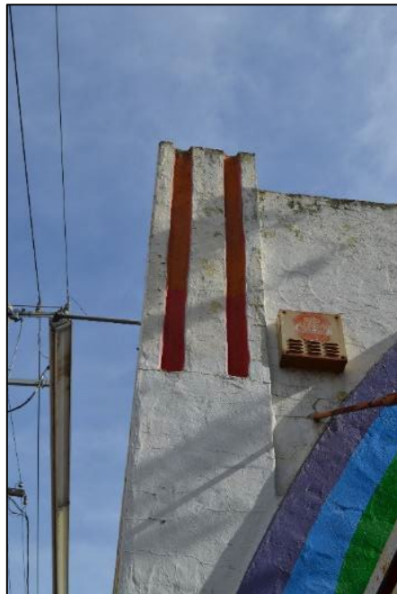
Detail of the fluted pier at the northwest corner of 2455 Telegraph Avenue
