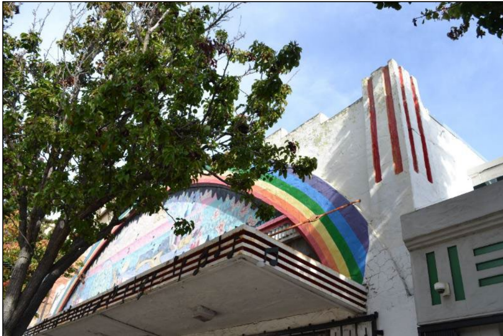
View of the marquee, arched frame, parapet, and corner pier at the front façade, viewed facing northeast
