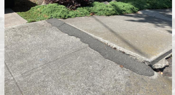
Before: Damaged sidewalks and long repair waitlist
