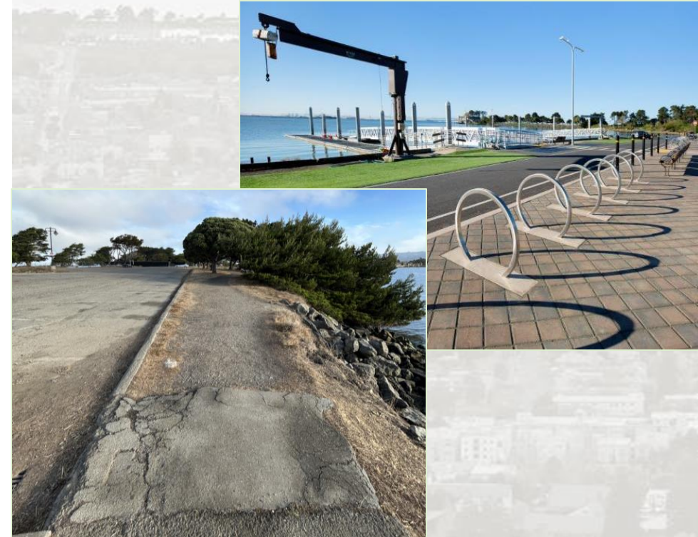
Above Images: Bay Trail showing pavement damage (bottom left) alongside sections that have received recent improvements (top right)
