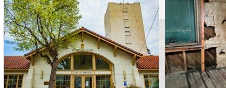
Before: Constrained, outdated training site, including water damage (top right image)
