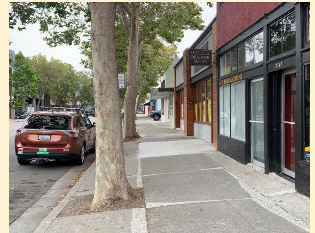
Sidewalks in many locations in need of maintenance
