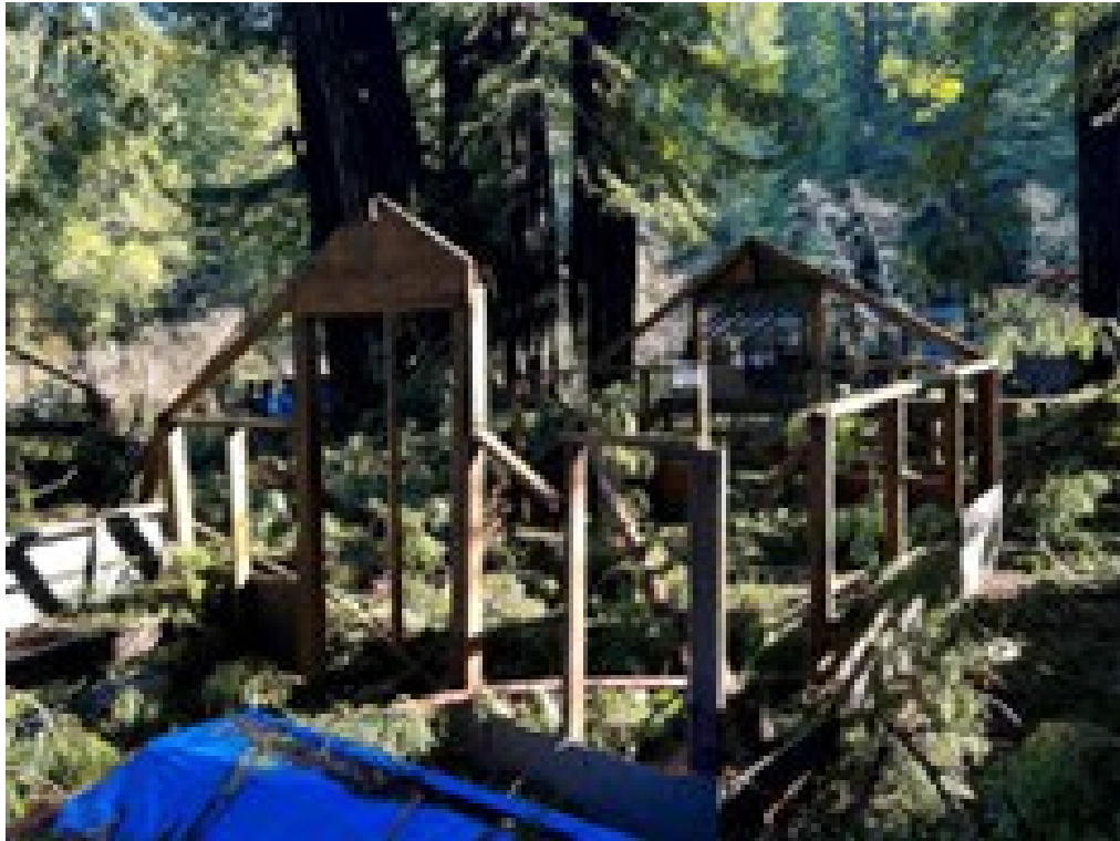
Cazadero Camp Storm Damage Recovery
