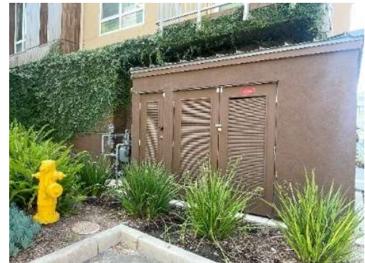
Figure 22. Utility Equipment Location Photo by AWP
