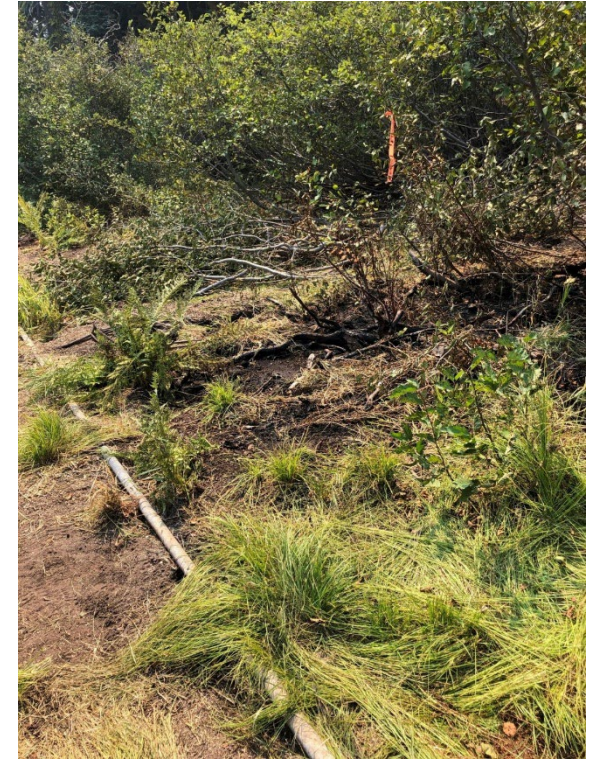
Echo Lake Water Intake Line
