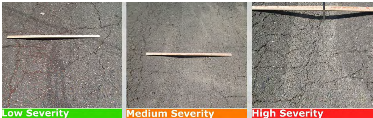
Image 6: Rutting and Depressions
