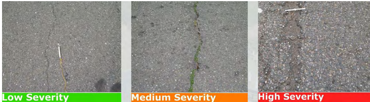
Image 4: Longitudinal and Transverse Cracking
