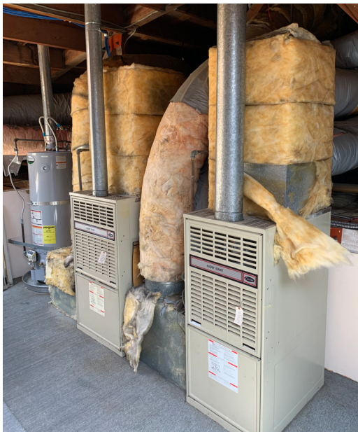
Figure 15: Furnaces at mezzanine floor.
