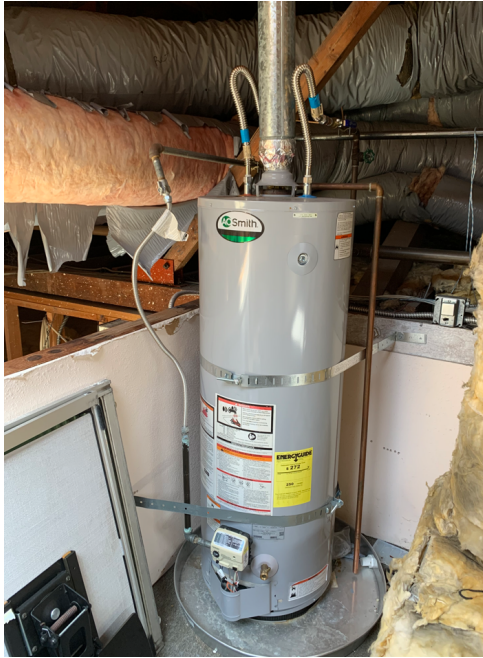
Figure 14: Restrained water heater at mezzanine floor
