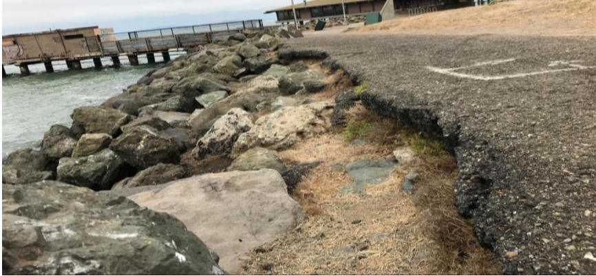
Before: Corroded, deteriorating seawall
