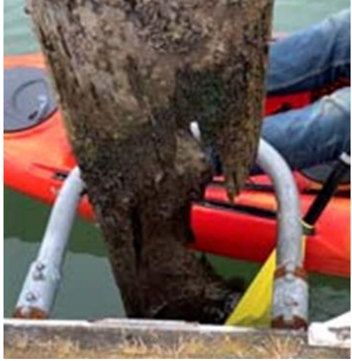
Before: Decayed timber piles
