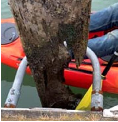
Before: Decayed timber piles
