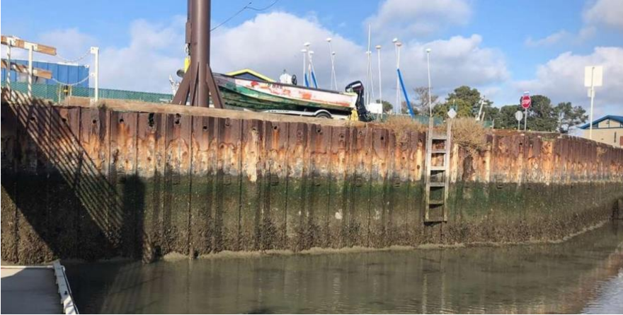
Before: Corroded, deteriorating seawall
