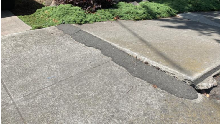
Before: Damaged sidewalks and long repair waitlist
