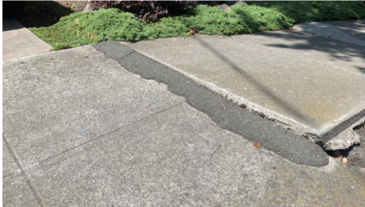
Before: Damaged sidewalks and long repair waitlist
