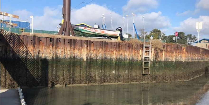
Before: Corroded, deteriorating seawall
