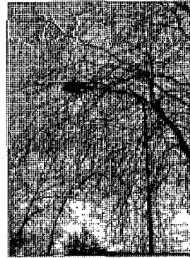
Figure 6: Light from this 'cobra-head' fixture is partially blocked by this street tree
