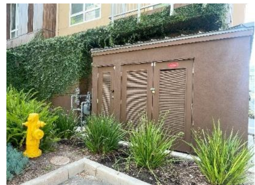
Figure 22. Utility Equipment Location Photo by AWP
