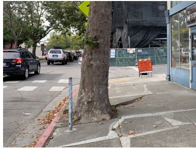
Figure 27. Many existing sidewalks are in poor condition.
