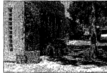
Figure 4: Planters and poorly maintained plantings are encroaching on the public right-of-way
