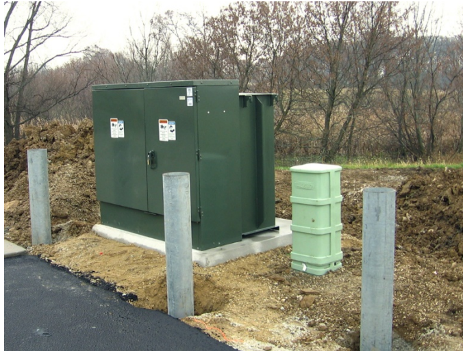
Figure 1. Pad-mounted (above-grade) transformer installed on a concrete pad with protective bollards. The equipment is visible and requires a dedicated footprint and clear working space for access and maintenance.
