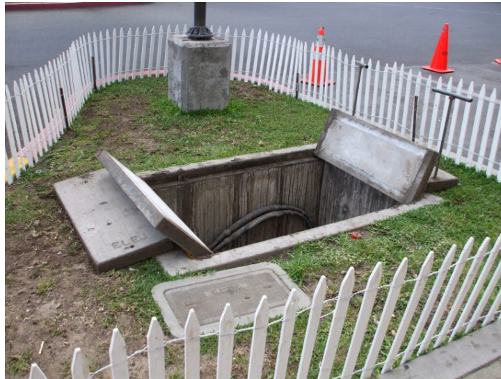
Figure 2. Underground transformer located on private property.
