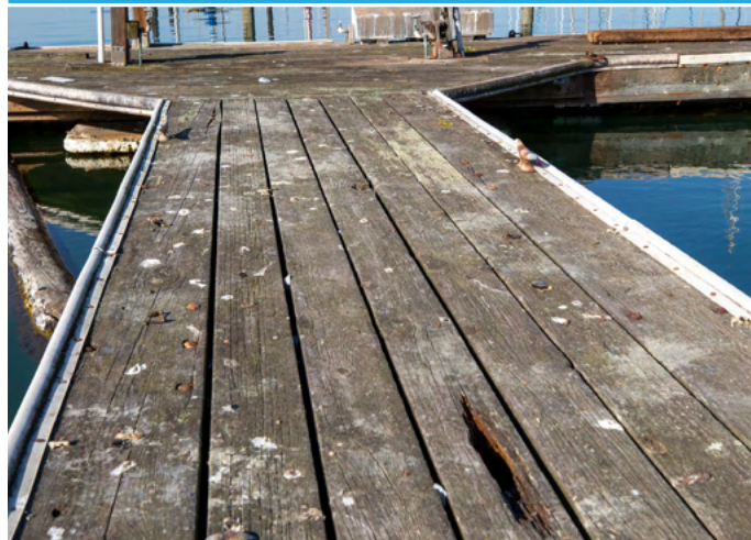
Deteriorated Marina Dock
