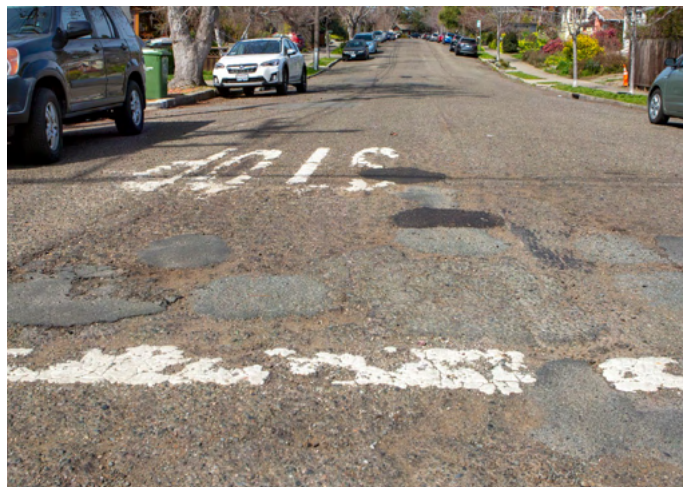
Street Pavement Damage
