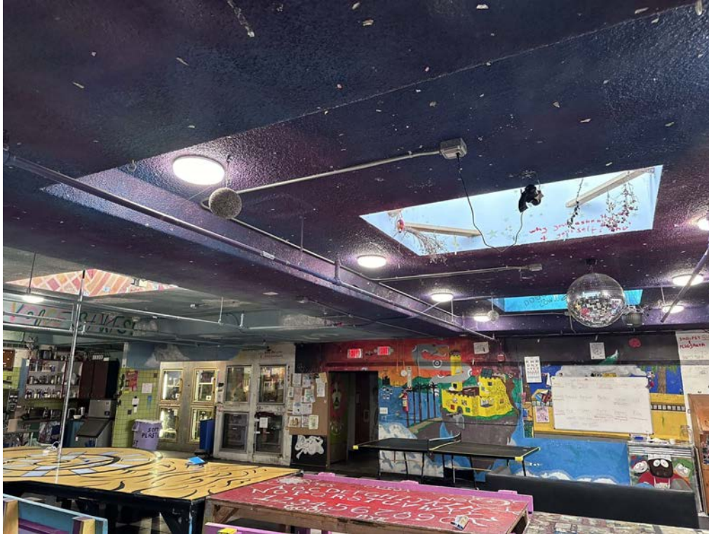
Images of broken skylights in Casa Zimbabwe common areas.
