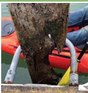
Before: Decayed timber piles
