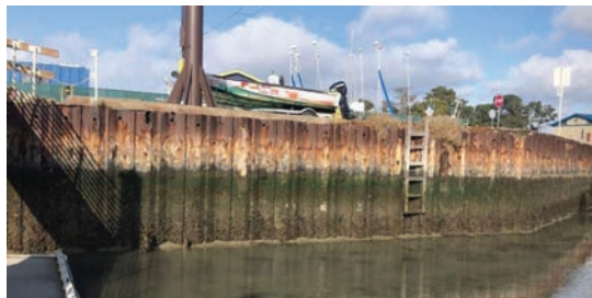
Before: Corroded, deteriorating seawall
