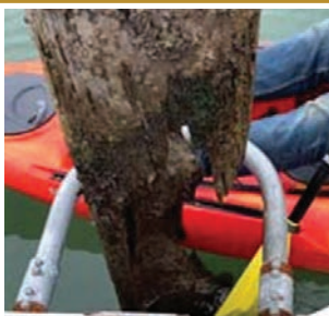
Before: Decayed timber piles
