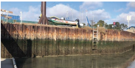
Before: Corroded, deteriorating seawall
