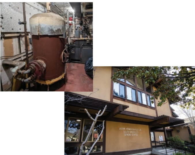
Before: Existing boiler and water heating system (electric heat pump replacement underway in 2026). South Berkeley Senior Center exterior.
