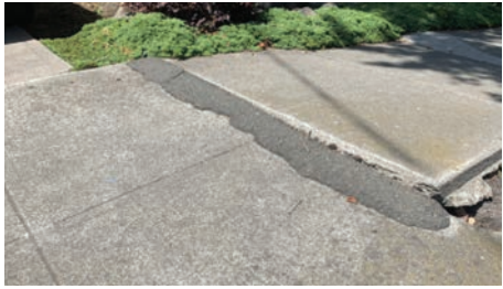
Before: Damaged sidewalks and long repair waitlist
