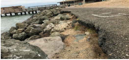
Before: Corroded, deteriorating seawall
