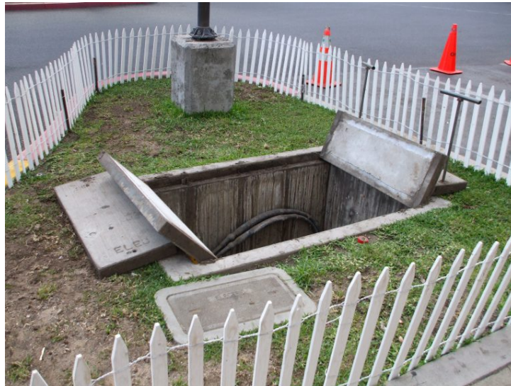
Figure 2. Underground transformer located on private property.
