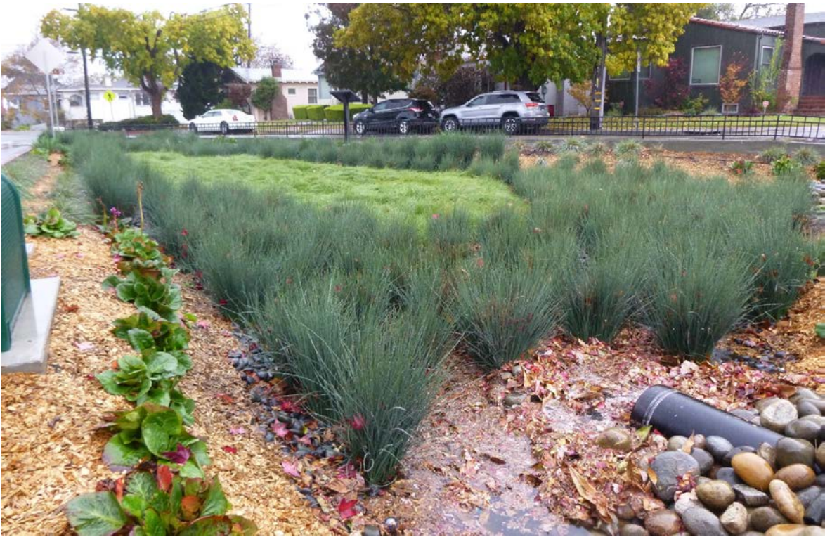
Figure 5 – A large concrete traffic island/median was reconstructed with a bioretention facility at Rose and Hopkins Streets.
