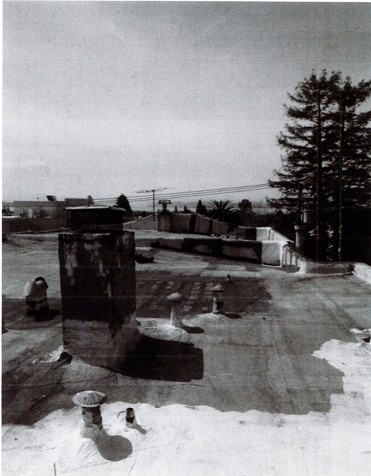
Foreground – chimney for Apt F facing west (A and B chimneys in the background)
