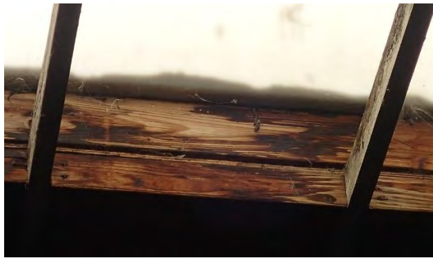
Figure 25: Concrete Building, Water Stains and Check on Beam
