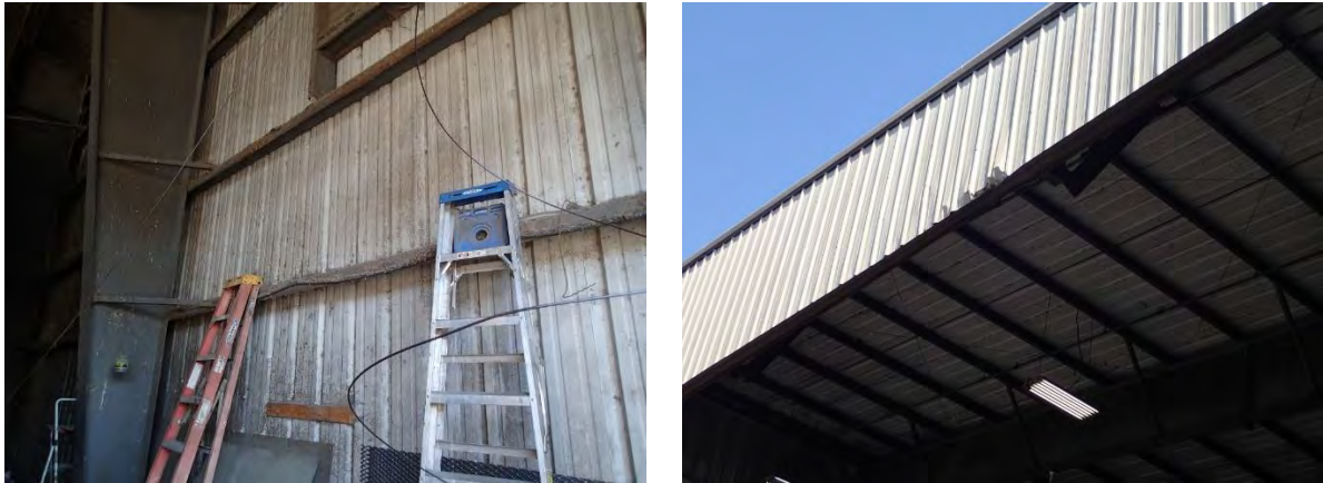
Figure 32 & 33: MRF, Rusted Secondary Members (Left) & MRF, Minor Damage on Siding (Right)
