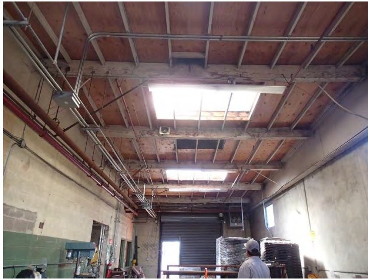
Figure 26: Concrete Building, Sagging Roof Beams, Damaged Beam Flange and Buckled Flange Brace
