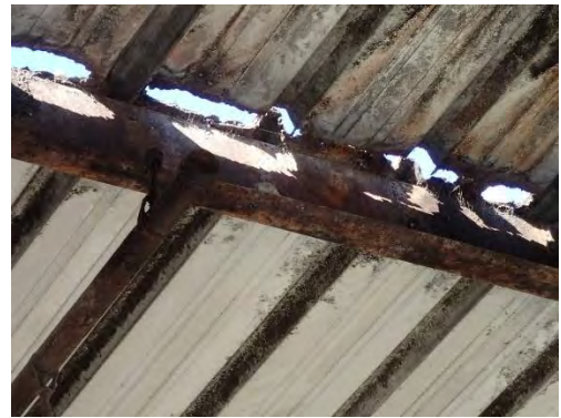
Figure 6: TS Corroded Roof Deck & Roof Purlins
