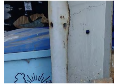
Figure 11: Storage Shed, Warped Column Flange
