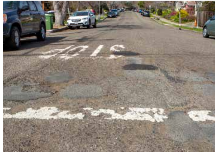
Street Pavement Damage
