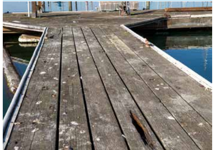
Deteriorated Marina Dock
