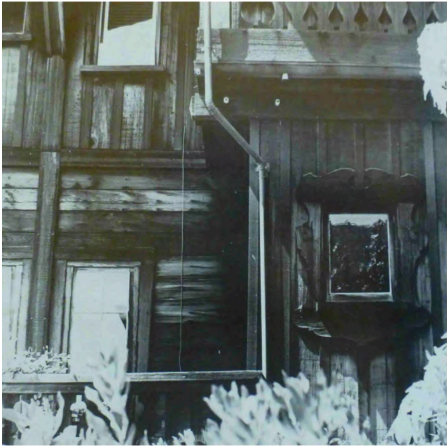
(At left. 1970s photograph of south facade, showing deteriorated horizontal board siding at first floor level, original French doors from living room to balcony at left, and original scroll-sawn wooden surround for vestibule window, at right. Source: Freudenheim.)
