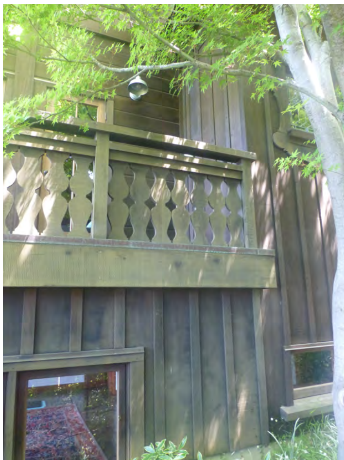
(At left. View of south wall, showing lower balcony and how it dead-ends into vestibule wall; one of the French doors to balcony from living room; change in siding from horizontal boards to vertical boards and battens at main level. Photo S. Finacom, 2021.)
