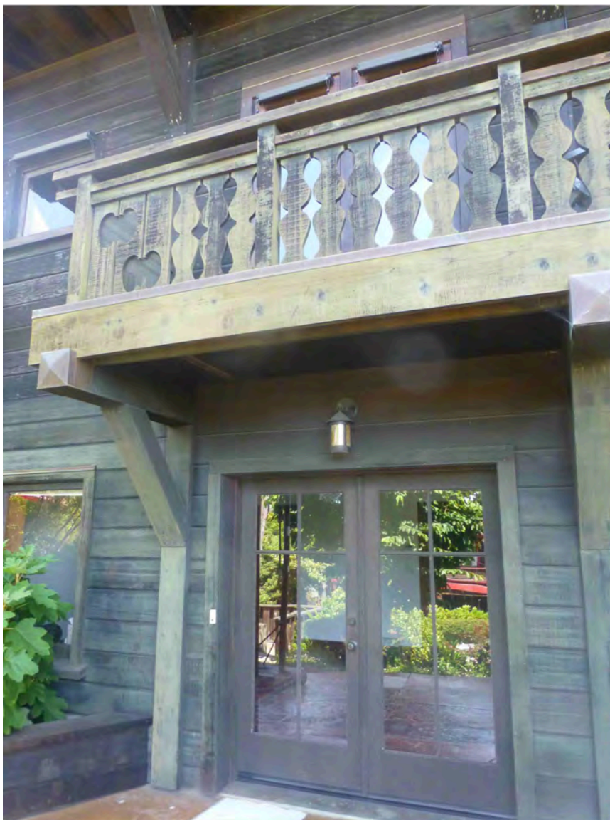
(At left, detail of basement level with newer French doors. Photo S. Finacom, 2021)
