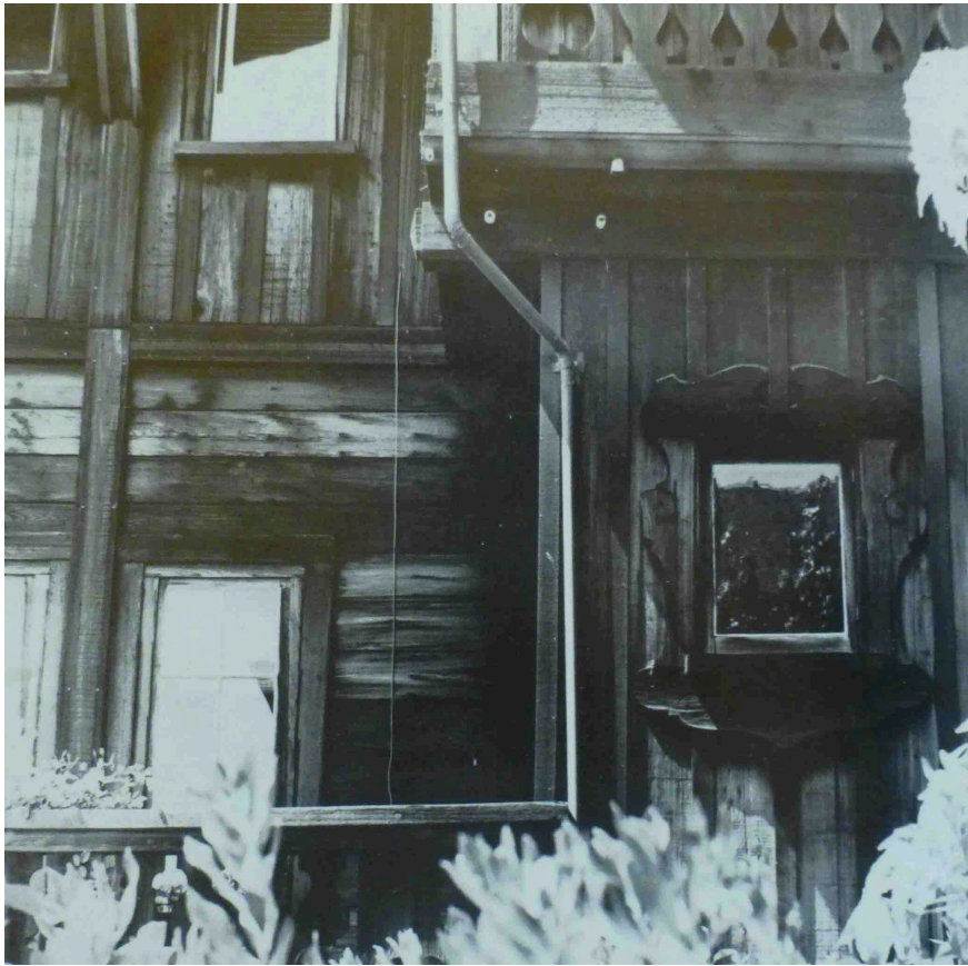
(At left. 1970s photograph of south facade, showing deteriorated horizontal board siding at first floor level, original French doors from living room to balcony at left, and original scroll-sawn wooden surround for vestibule window, at right. Source: Freudenheim.)
