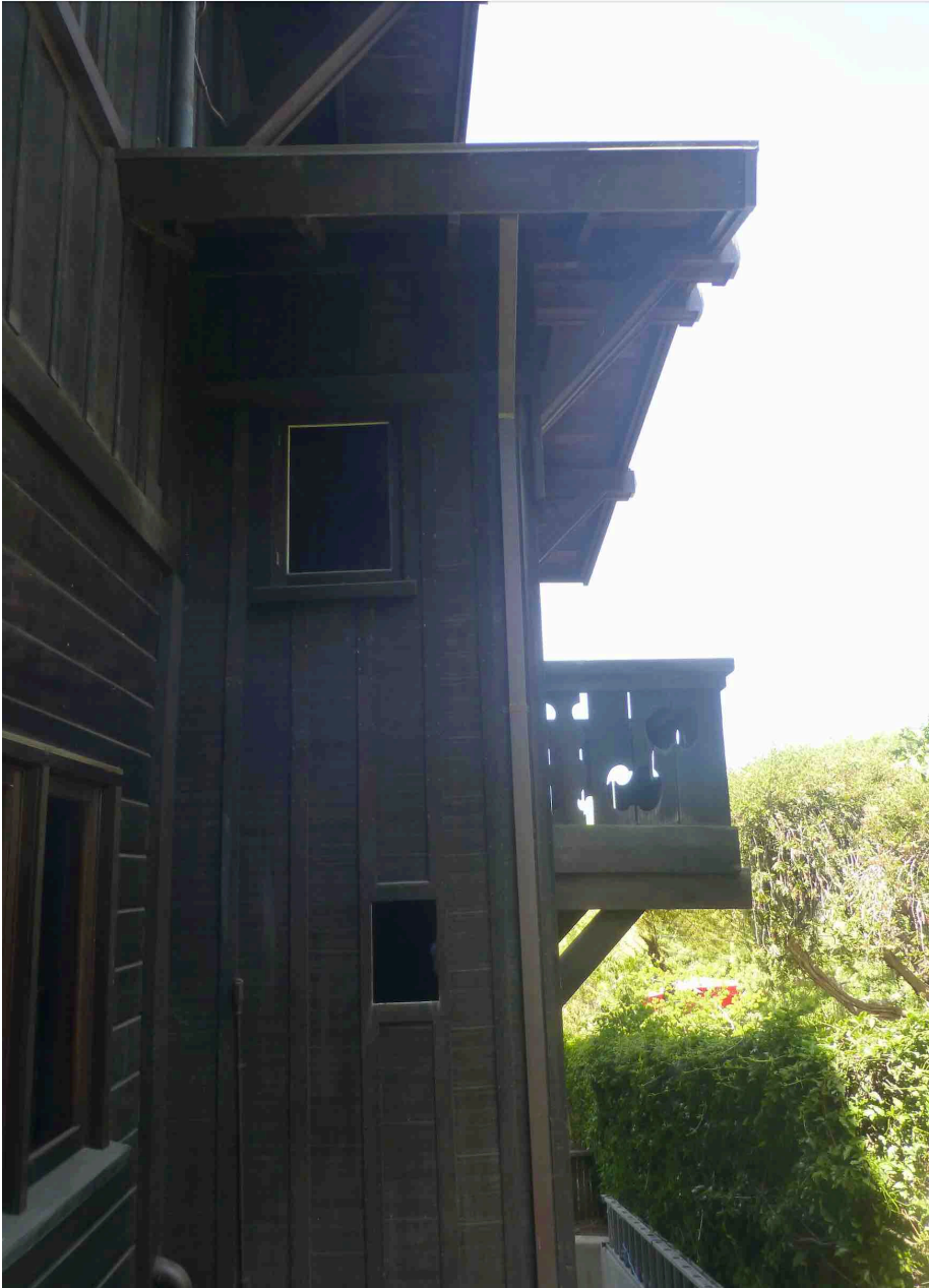
(At left, looking west, along the north wall of the original house, showing the one and a half story board and batten bay that contains the stairwell. The “Juliet” balcony is on the right, and there is a small hipped roof over the projecting bay. Photo S. Finacom, 2021.)
