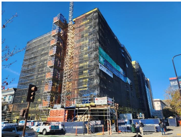
Figure 12: Phase two of Identity Logan Park at 2370 Shattuck Avenue, an eight-story mixed-use multifamily building under construction. Looking northwest.
