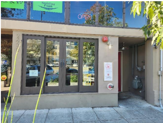
Figure 4: Detail of north side of east façade, showing hinged storefront window fixture and emergency exit recess. Looking west.
