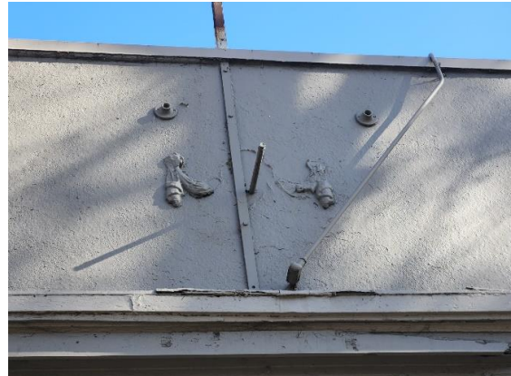
Figure 5: Detail of damaged cartouche above south storefront at west façade. Looking east.
