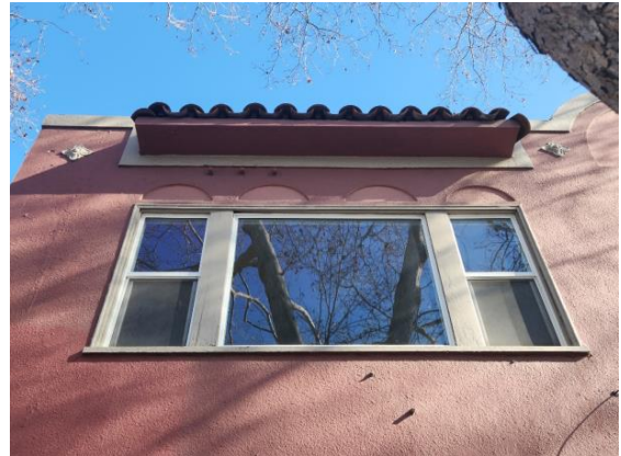
Figure 5: Second story windows and ornaments over north storefront on the west façade. Looking east.
