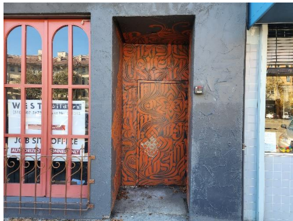
Figure 5: Detail of emergency exit at north end of east façade. Looking west.
