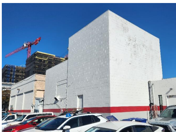
Figure 8: View of southwest corner of subject building, showing one-story and two-story concrete masonry unit additions. Looking northeast.
