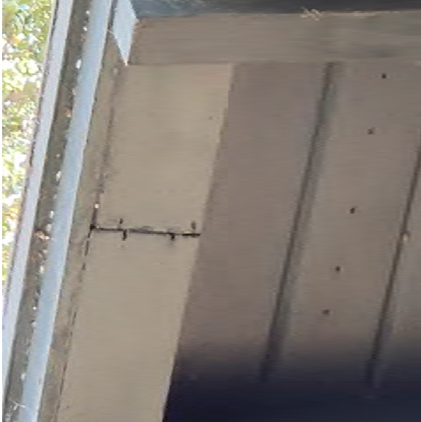
Dry rot at eave, fascia, and integral wood gutter (typ.).
