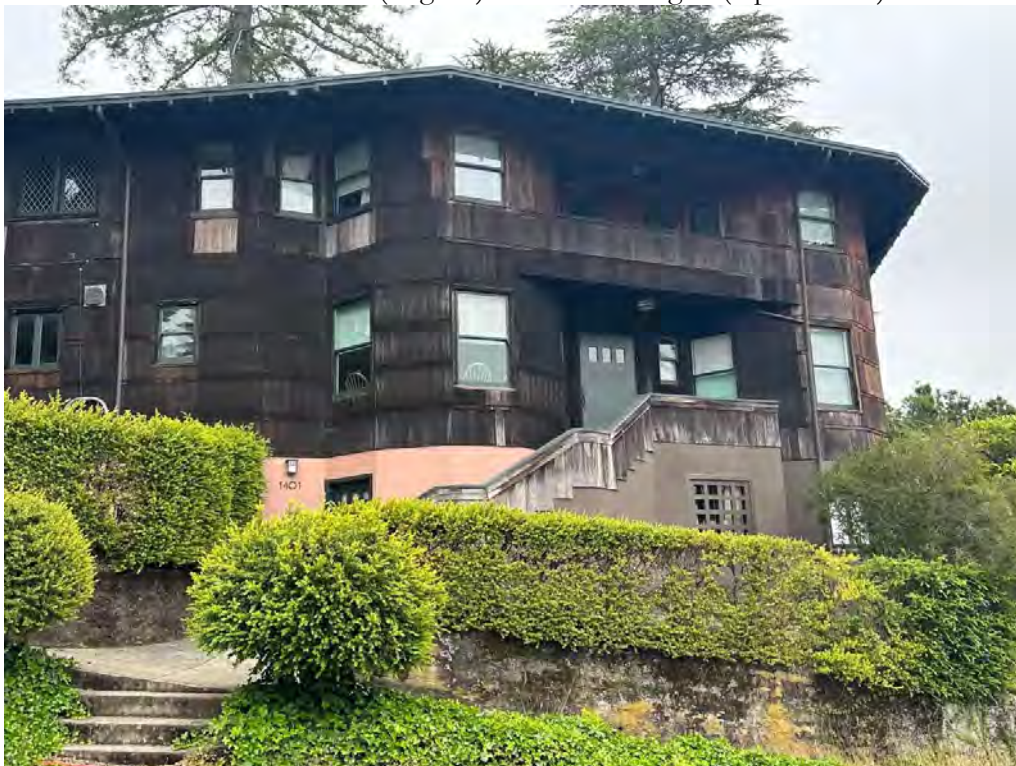
Circled windows proposed for replacement. Dry rot on most trim at sills and sashes.
