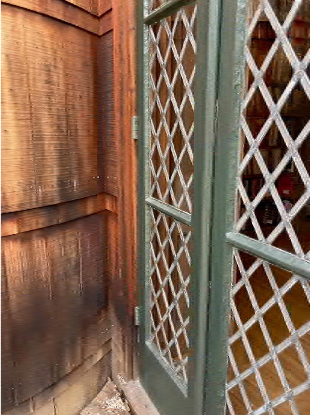
Dry rot at sill.
