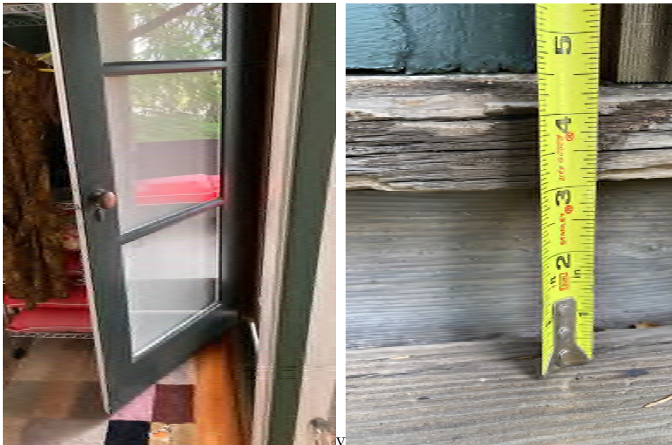
Dry rot at sills
