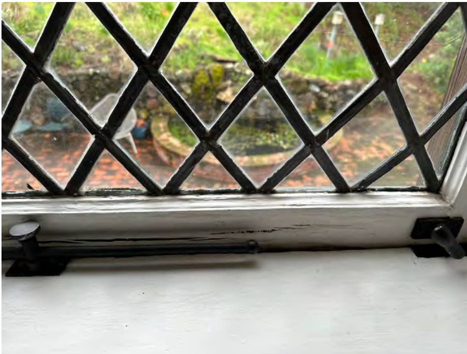
View of leaded glass windows on south façade. Note leaded glass pulling away from wood sashes.
