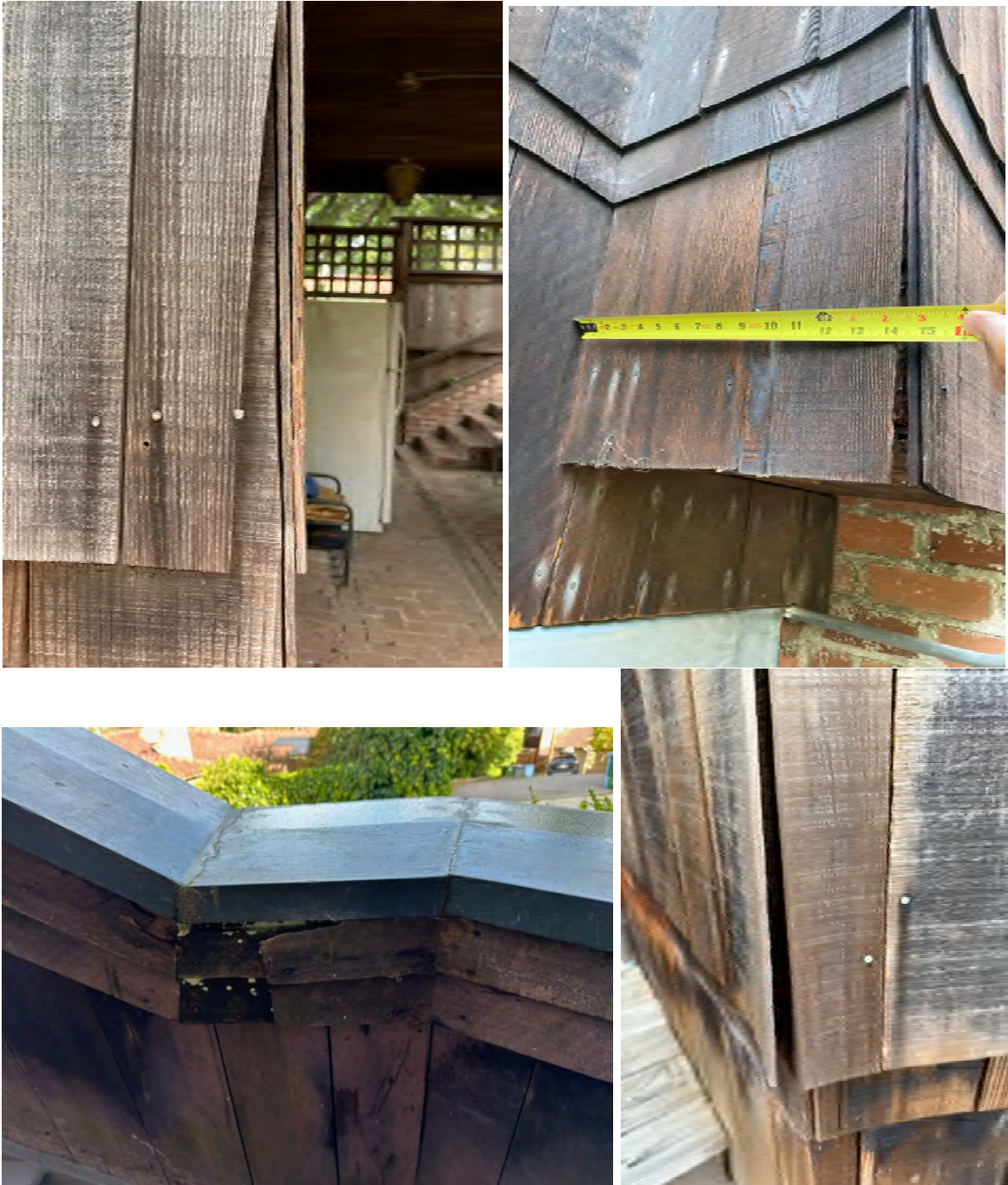
Shakes in various state of disrepair, age.
