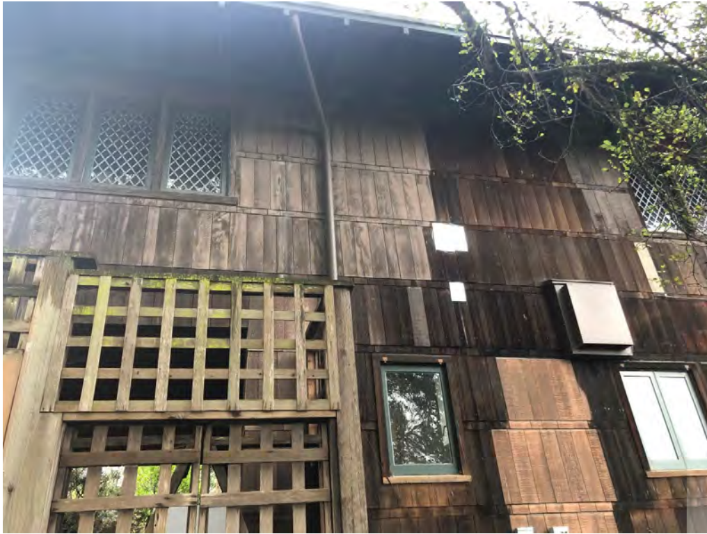
Patchwork of redwood shakes (original) and cedar shingles (replacement).
