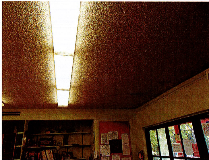
Photo 2 Spray-on acoustical texture over concrete ceiling contains up to 25% chrysotile asbestos and fluorescent light fixtures with assumed PCB ballast.
