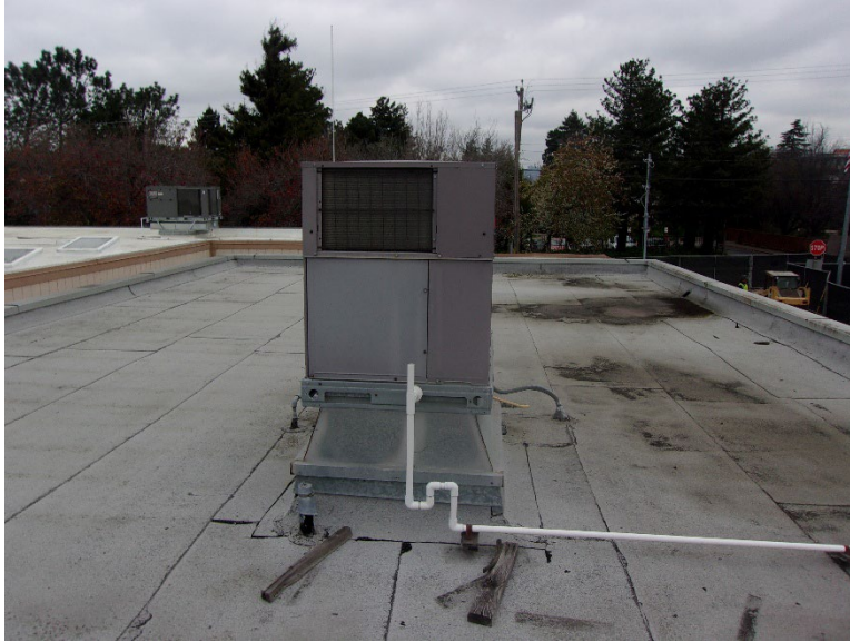
Photo 3 HVAC unit with Freon.
