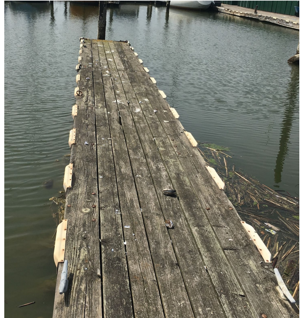
Deteriorated Finger Dock and Piling – Needs Replacement
