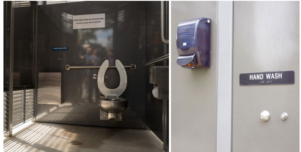
Image A22 and A23: Portland Loo at a sidewalk (inside and outside)
