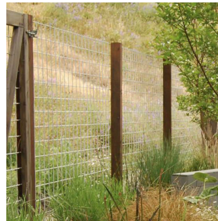
WIRE MESH FENCING
