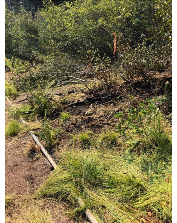
Echo Lake Water Intake Line
